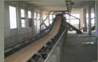
Transfer to Silo
