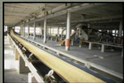
Transfer to Silo
